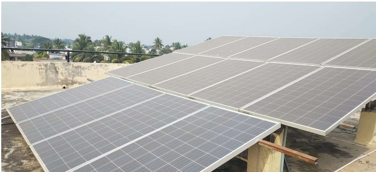
Figure 3 Roof-Top Solar System
